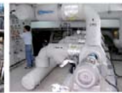
Chiller Pipes and Pumps
