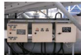
Water Tower Automatic Water Treatment
