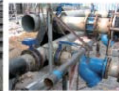
Valves and Condensing Pipe Connection
