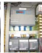
DDC Control Panel Inside
