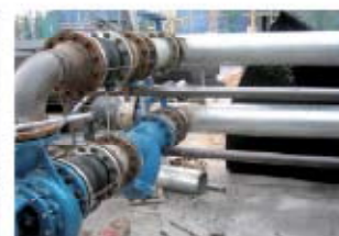
Condensing Pipe Connection
