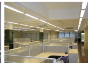
Office with VRV Indoor Units
