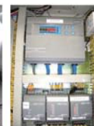
DDC Control Panel Inside
