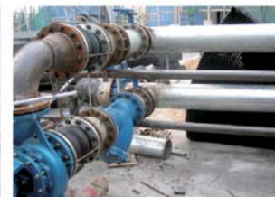
Condensing Pipe Connection
