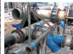
Valves and Condensing Pipe Connection
