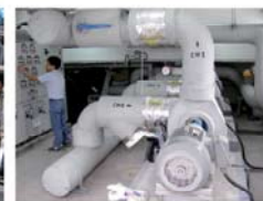
Chiller Pipes and Pumps
