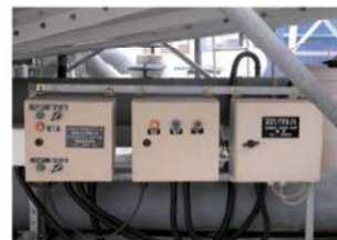
Water Tower Automatic Water Treatment
